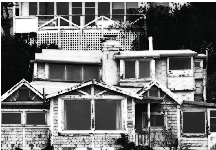
Cottage #11 on the North Beach is in dire need of restoration.
